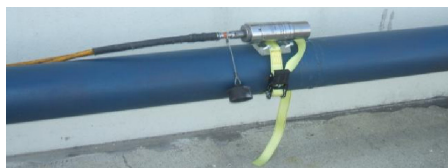
Figure 1: Sentinel's Model 989 SCAR exposure device applied to 6" pipe for uses in weld quality radiograph
