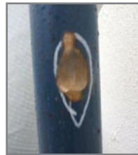
Manufactured defect in 2" piping
